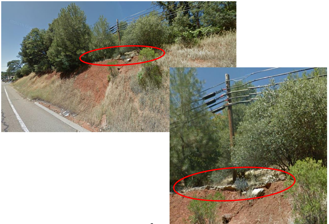
Figure 2. Paving Remnants as Seen From Placerville Drive (Source: Google Maps)
